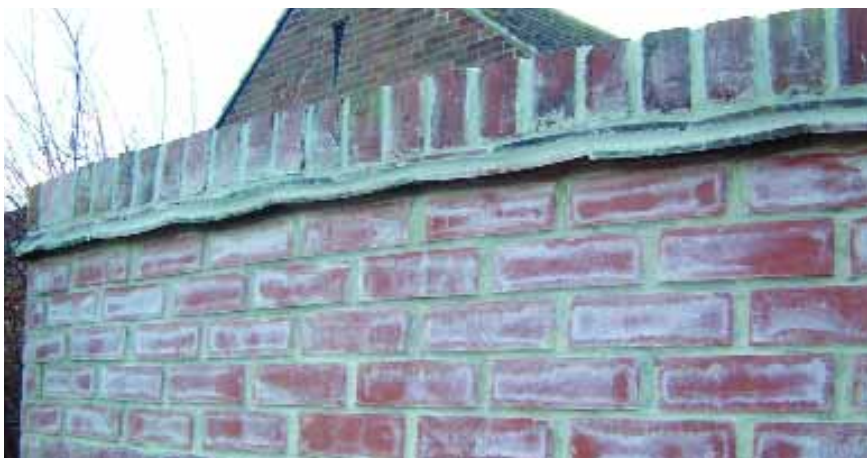
Brickwork with evidence of efflorescence
