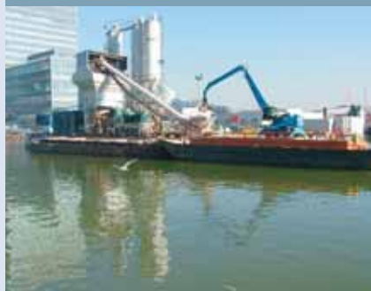
Hanson have found an innovative solution to avoiding the capital's congested streets whilst delivering ready-mixed concrete for high-rise developments in Canary Wharf. This floating plant at West India Docks is itself supplied by barge, significantly reducing the number of aggregate lorry journeys to site.
